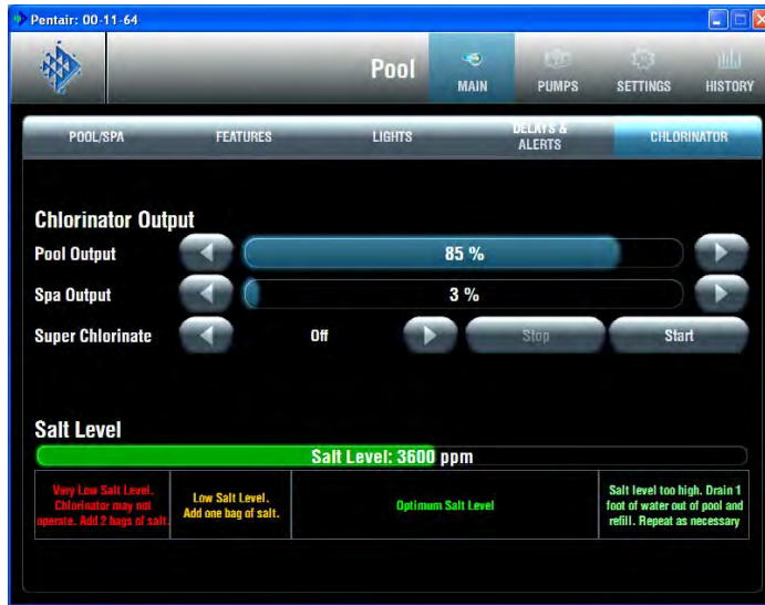
Chlorinator (IntelliChlor) screen
